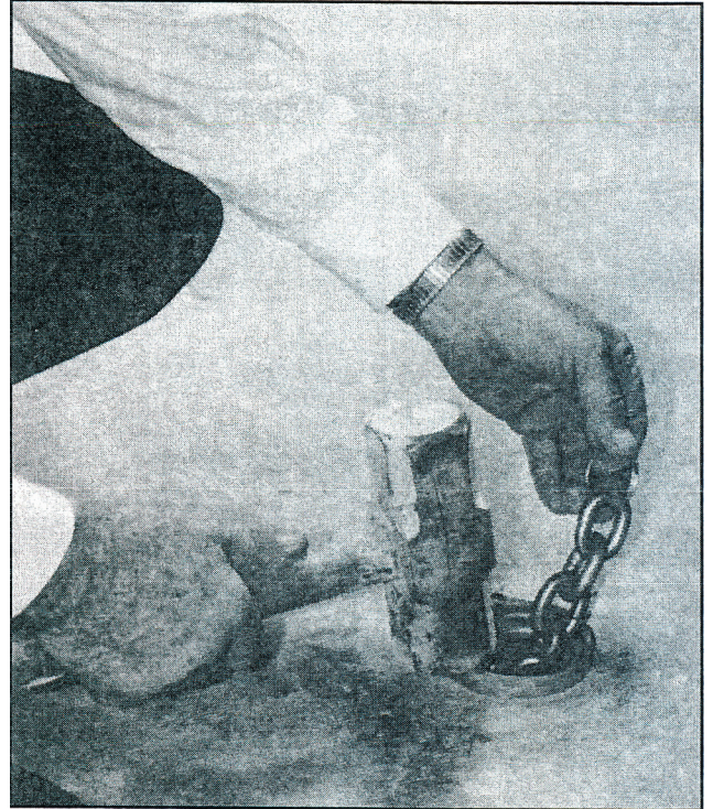
Use a small sledge hammer to tap rim of anchor sleeve until it is flush with floor.
