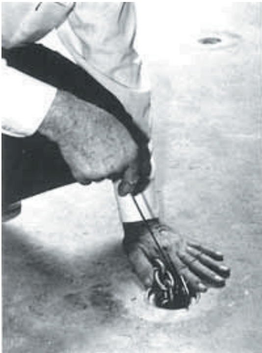
Pull chain retaining wedge completely out of T-slot on anchor expander and remove from floor anchor.
